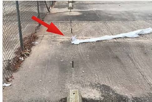
Example of missing parking curbs.
