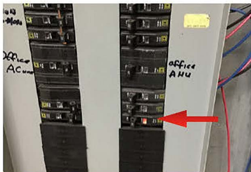
Tripped breaker in panel F
