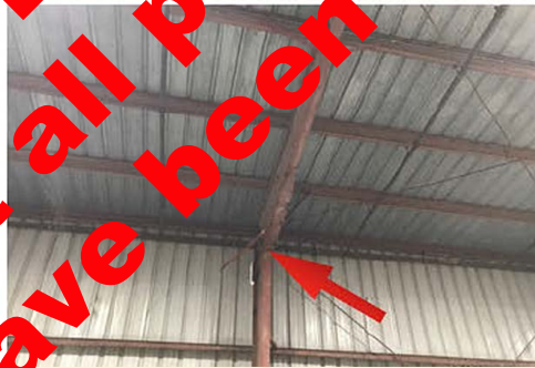
Another loose truss framing
