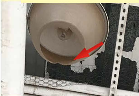
Exterior light with broken cover.
