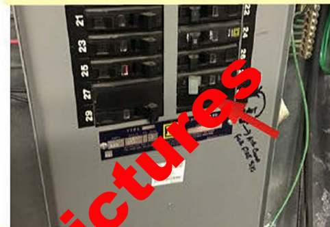
Lock out needed on fire suppression breaker
