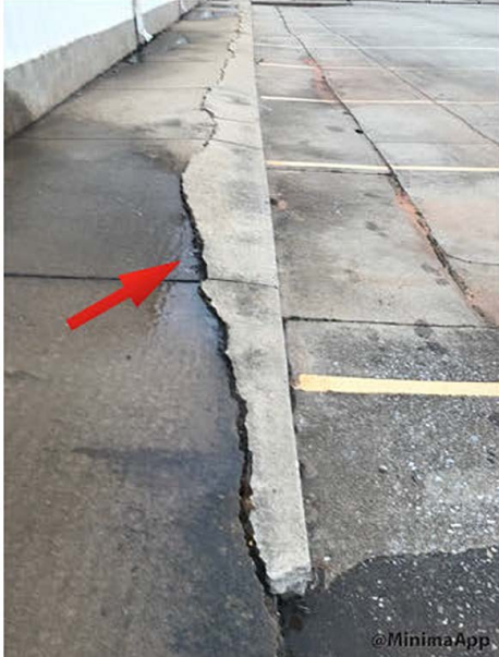
Street creep on the South side of the main building.
