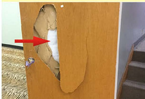
Example of damaged door, SW of entry doors
