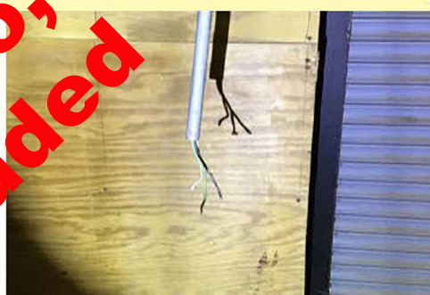
Loose wires in suite F
