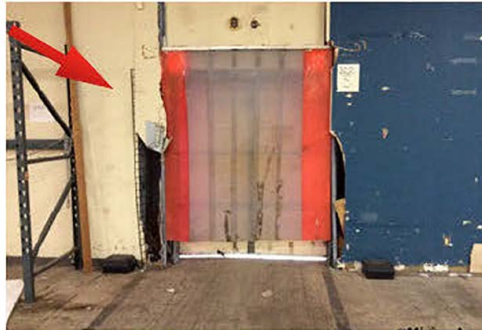
Damaged wall around suite b overhead door.
