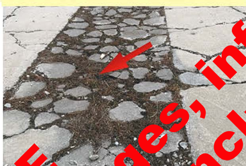
Example of damaged concrete in parking lot
