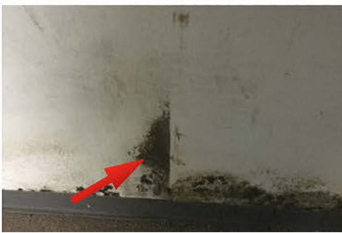
Mildew like substance SW room of entry door
