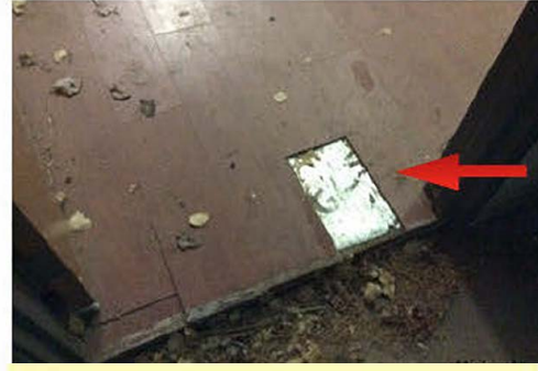
Laminate floor missing and damaged in suite G.
