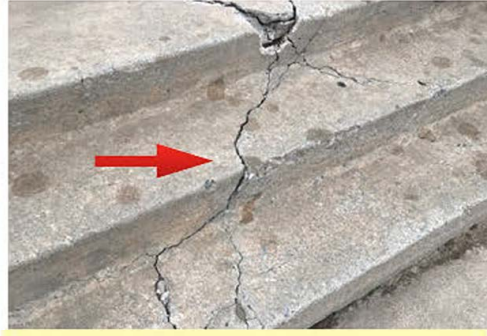
Example of damaged stairs.
