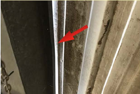
West side by dock door - metal siding not attached & allowing
