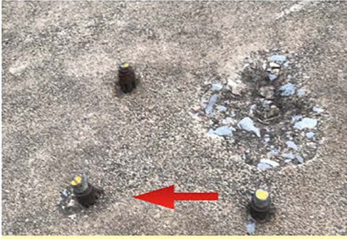
Example of a trip hazard, rebar was not cut flush with the ground.
