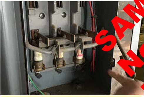
Shutoff box not being used outside of suite F
