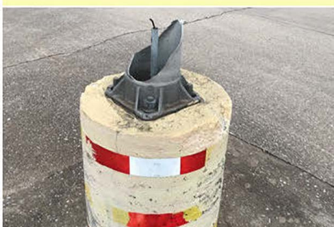
Light pole that is broken off at the base.
