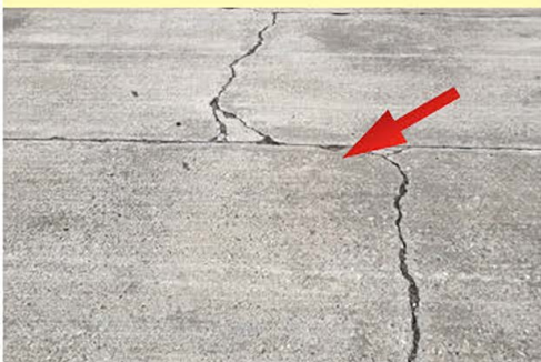
Example of damaged parking lot.
