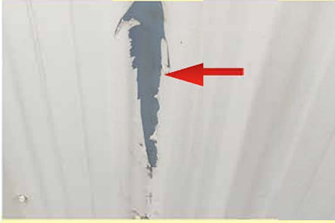
Example of damaged exterior wall that needs paint.
