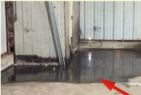
Flooding and mildew like substance in suite G
