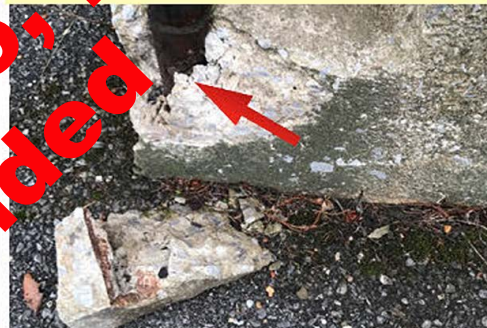
Example of concrete corner pop
