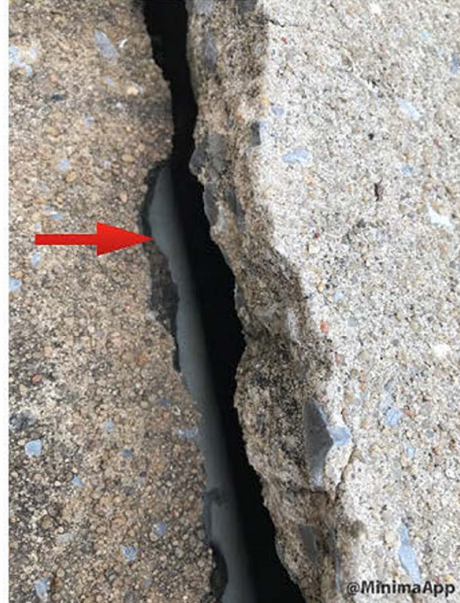
Close up view of the street creep on the South side of the building.
