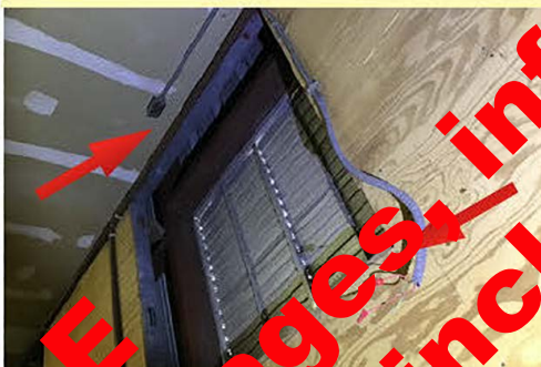
Loose wires and missing cover in suite F
