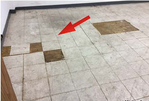
Vinyl floor tiles missing in bathroom in suite G.
