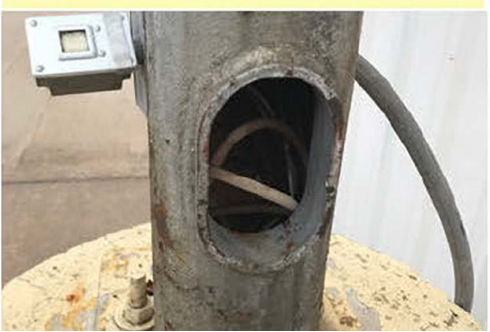
Missing access panel on exterior light pole.
