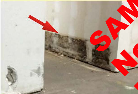
Example of mildew like substance in suite G.
