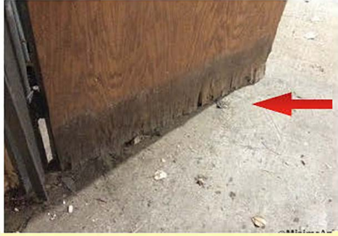
Door to warehouse in suite G delaminated.
