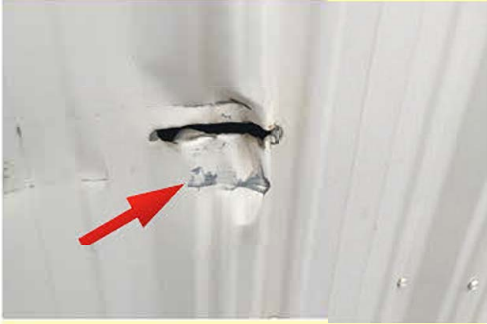
Example of puncture in exterior wall.
