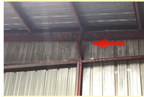
More damaged framing on the N. Wall
