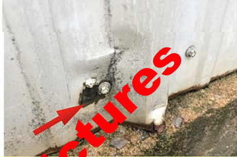
Example of dented exterior siding
