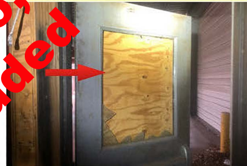
Boarded up, broken window in exterior door of suite F.
