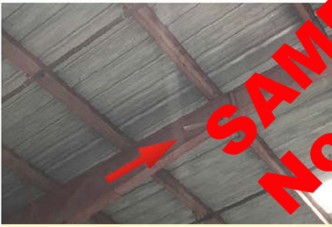
Loose truss anchor for roof framing
