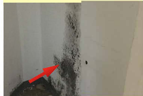
Mildew like substance SW of main entry doors
