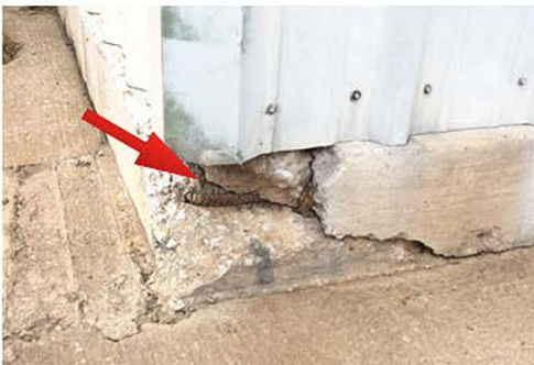
Foundation corner pop with exposed rebar on warehouse
