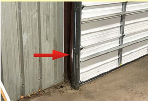
Damaged framing by S. Overhead door of warehouse
