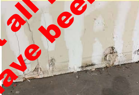
Example of drywall damage in Suite G.
