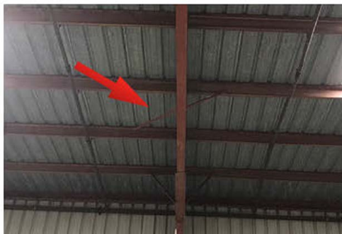
Loose truss anchor for roof framing
