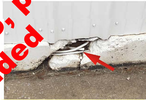
Rebar exposed on warehouse stem wall
