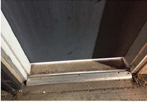
Suite G exterior door not weather tight.
