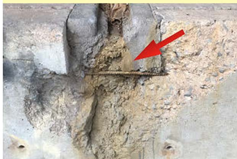
Example of damaged concrete.
